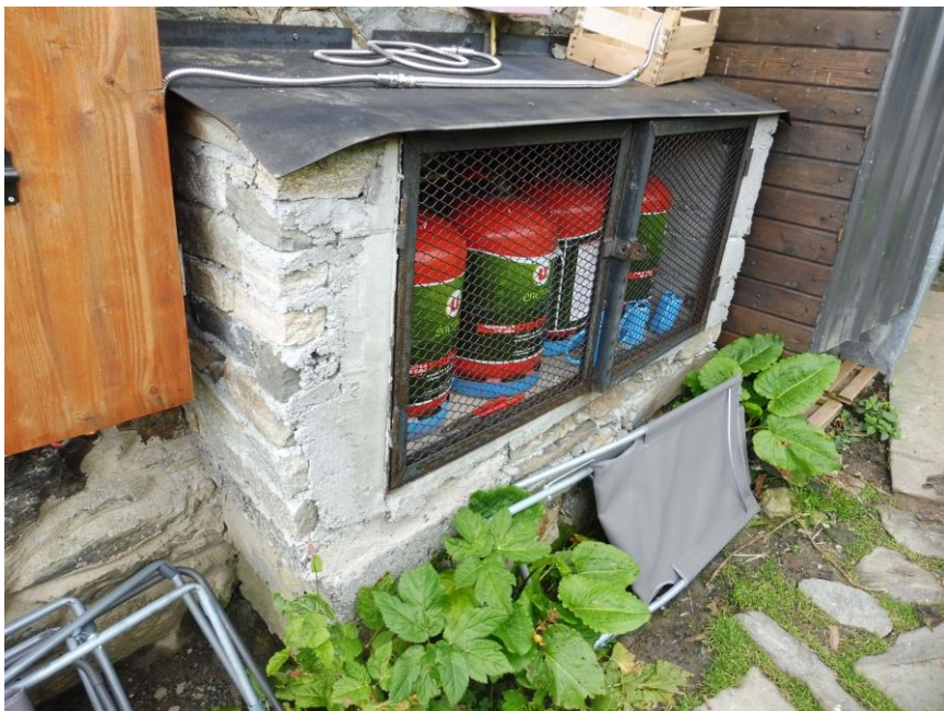
Stockage gaz (4 x P13)
